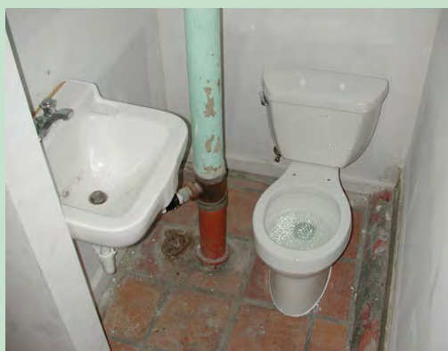
A basin and toilet.
